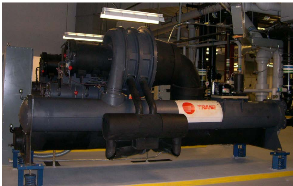
Central Cooling System Chiller 200-250 hp compressors
