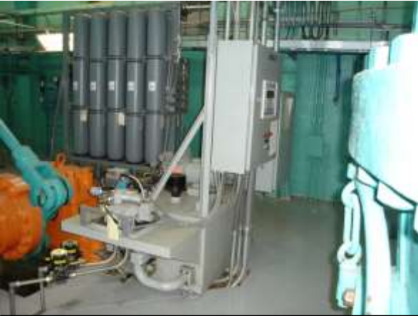
Hydro Governor for Servicing
