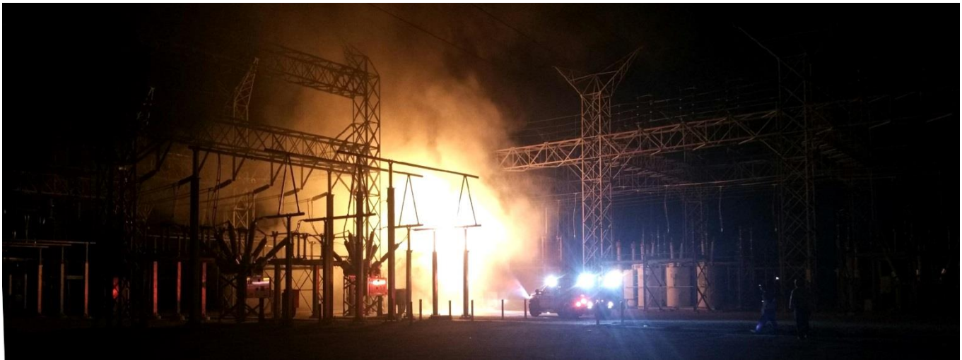
Photo credit Georgia Power
