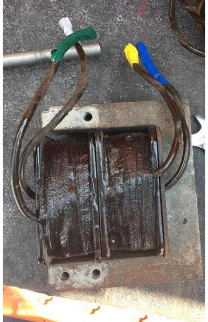
Figure 4: Burned Trip Coils
