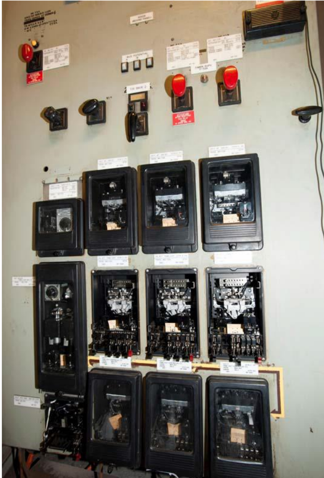
Figure 3: Relay Panel Under Test Following the Event (87N In Lower Left Hand Corner)
