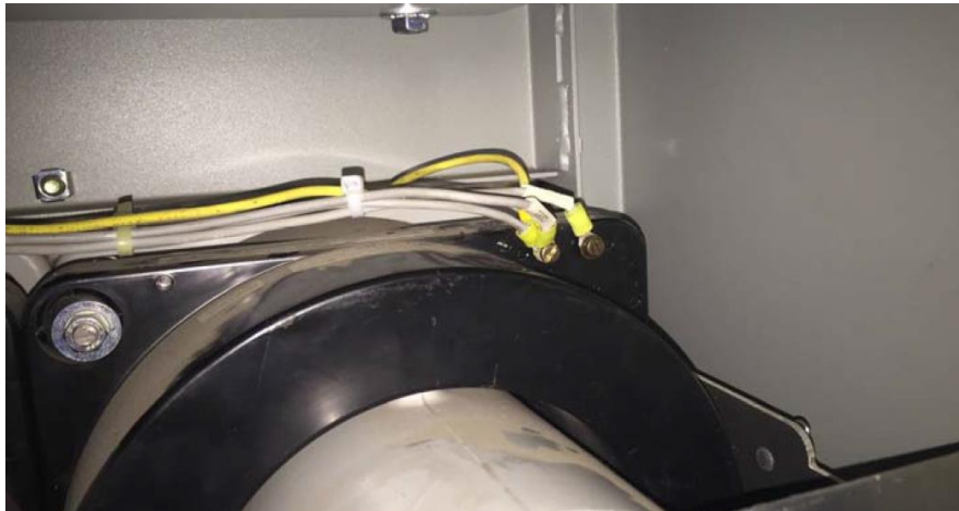
Figure 5: Added Neutral CT Connection to Complete 87N Circuit Post-Event
