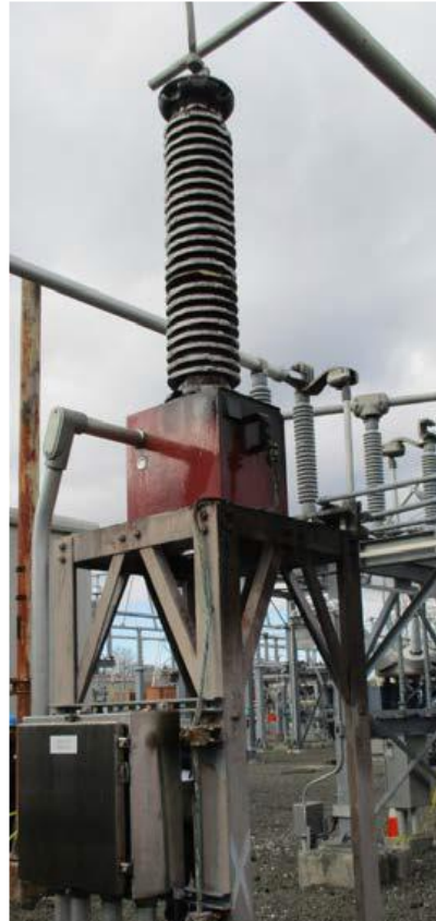
Figure 5: Damaged B Phase CCPD
