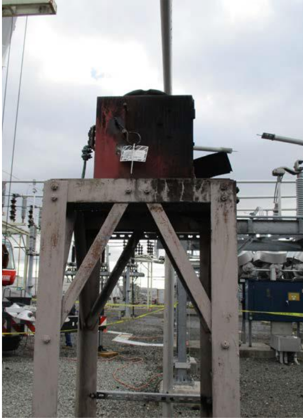
Figure 4: Failed C Phase CCPD
