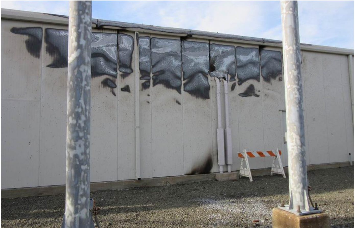
Figure 7: Exterior of Relay House Singed by Protracted Fault
