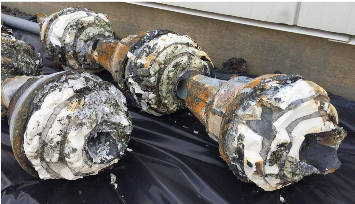
Figure 6: Remnants of Bus Insulators
