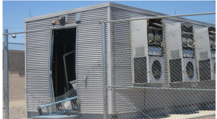
Figure 3: BESS Exterior after event (image credit: APS)
