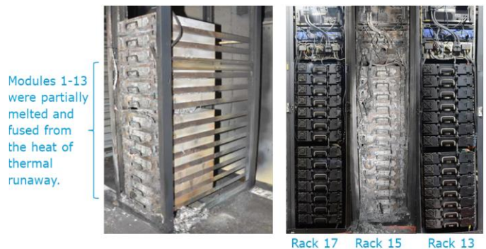
Figure 4: All modules in Rack 15 were severely damaged by thermal runaway while leaving nearby racks mostly intact (image credit: APS)
